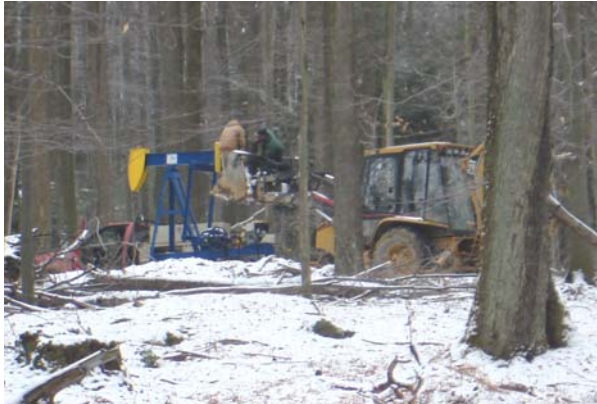
Installation of a new oil well along the Morrison Run trail, December 2006. Photo by Jessica Ley.
